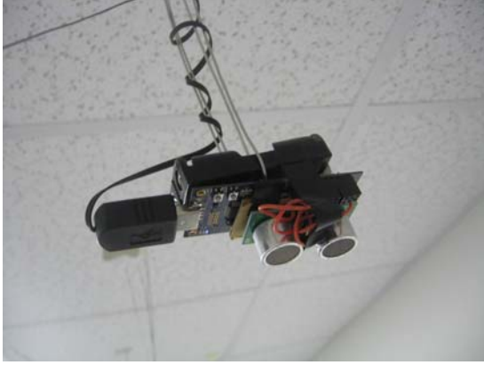
Fig. 1. Ceiling-mounted mote with attached ultrasound sensor
